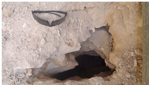
Figure 14. A void was encountered where the NP anomaly B is observed (see Figure 11). This void is enlarged to the north towards the McNeill High School and became a cave (Cave 5).
