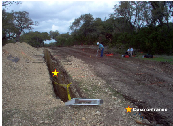
Figure 5. A picture showing the cave location along the trench. The cave is located 3.5 meter below the ground.
